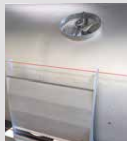
Inspection hatch for access on the air side of the membrane
